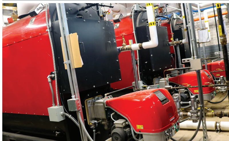
NEW BOILER AND INSULATED STEAM PIPES
