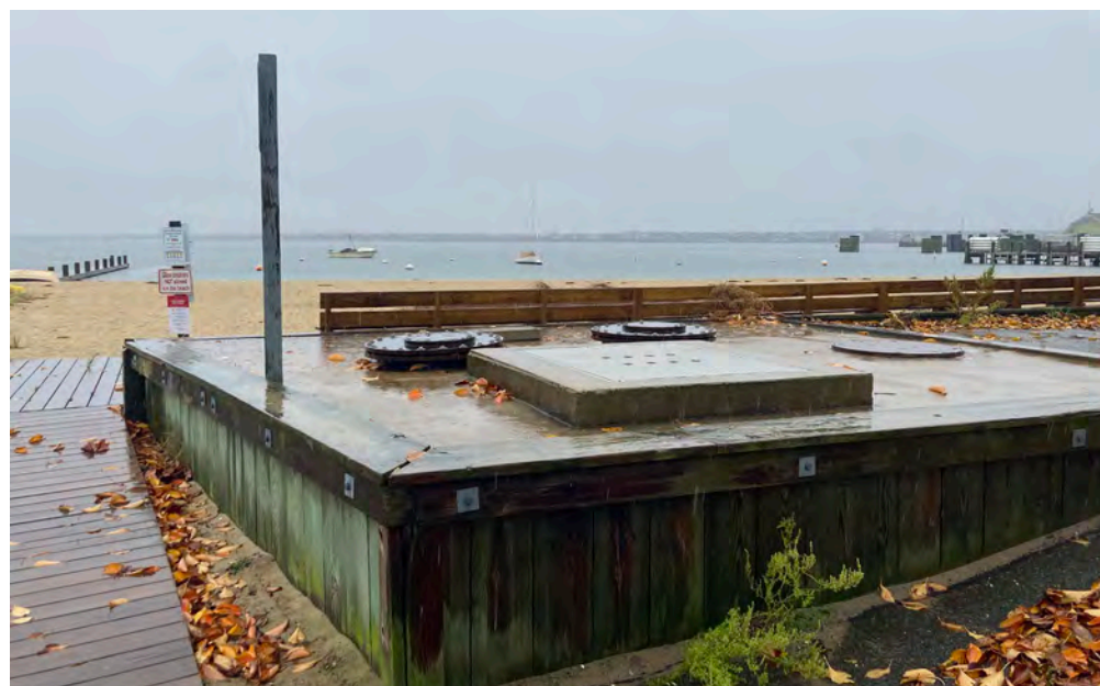
Children's Beach Pump Station, Trevor Johnson
