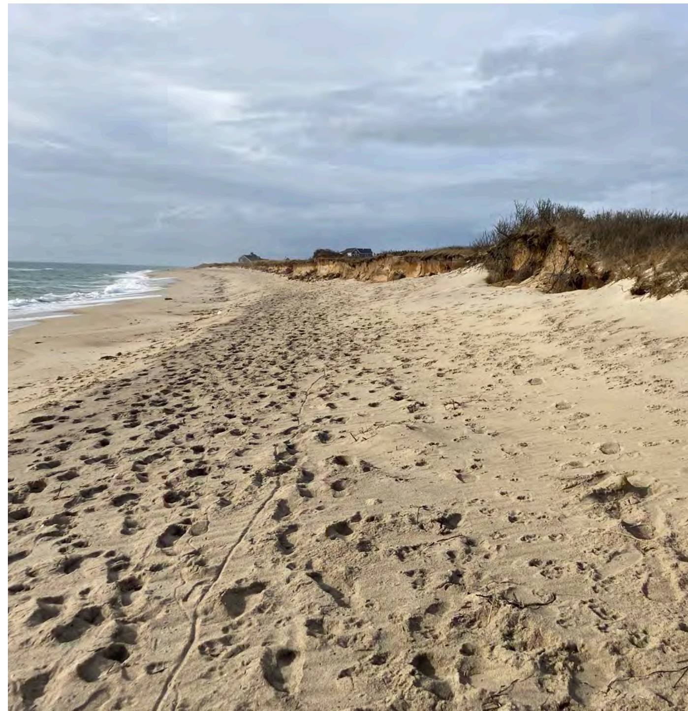
Coastal erosion (photo by Rennie Jones)
