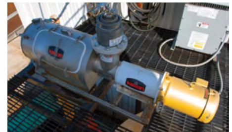
The CENTRI-SIFTER centrifugal sifter at the distillery runs at a higher voltage than normal in order to screen heavy, sludgy stillage.
