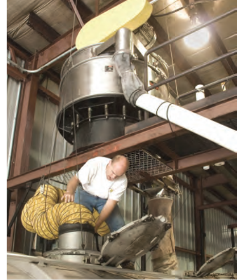
Each of the high-capacity discharge VIBROSCREEN units can screen up to 36 tons/hr, allowing trucks to be rapidly loaded with sugar.
