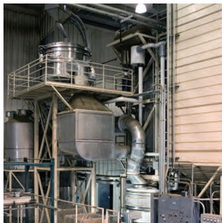
Almonds are conveyed from a holding tank (right) to a pasteurization tower (left of holding tank) from which they proceed to a fluid bed dryer (bottom) and then to a fluid bed cooler (top). Beneath the cooler is an equilibration tank where almonds achieve uniform temperature.
