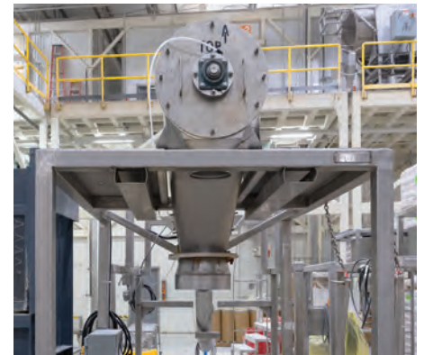
Centrifugal sifting maintains high throughput and product integrity at PacMoore's Mooresville, IN plant. Screened product gravity-discharges through a central chute.
