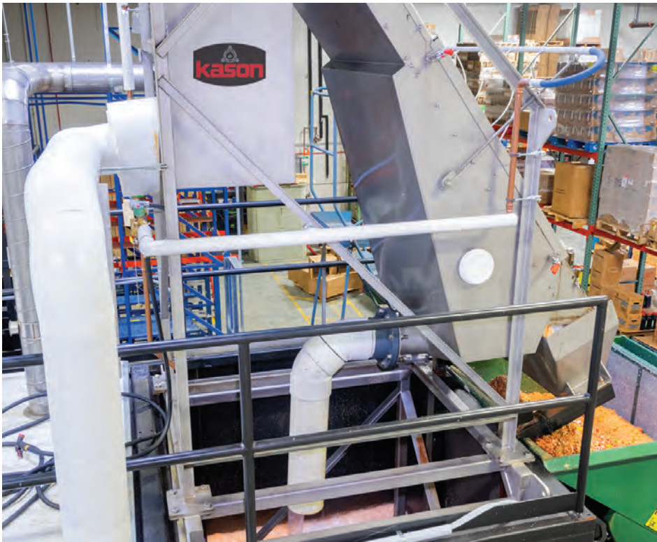
Wastewater is pumped onto the dewatering sieve which separates solids at high rates without the use of power.
