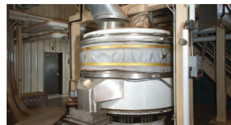
An 84 in. (2125 mm) diameter circular fluid bed dryer, clad with insulation blanket, dries almonds to moisture content between 4.5 and 5.5 percent. Throughput rate is 22,000 lb (9,979 kg/h) per hour.
