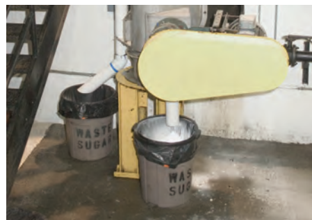
Oversize material falls through a 4 in. (102 mm) diameter chute and drops into a tailings bin.
