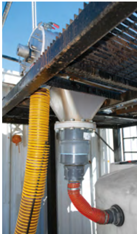
Oversized grain solids exit through downspouting into an enclosed container. Recovered liquid (sour mash) gravity feeds through the center discharge, is stored and added to subsequent fermentation batches.
