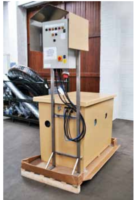
External Control Panel and Permeate Tank
