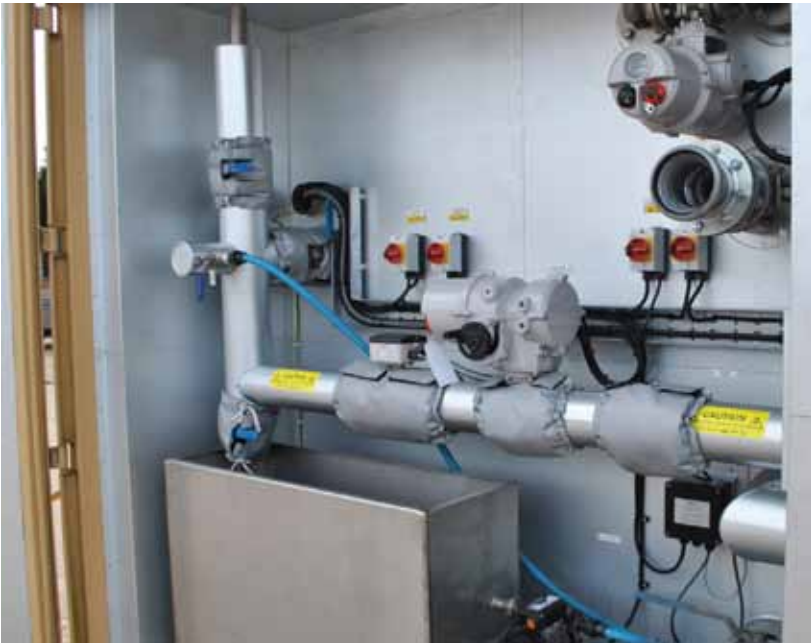
Built In Chemical Cleaning Plant Tank
