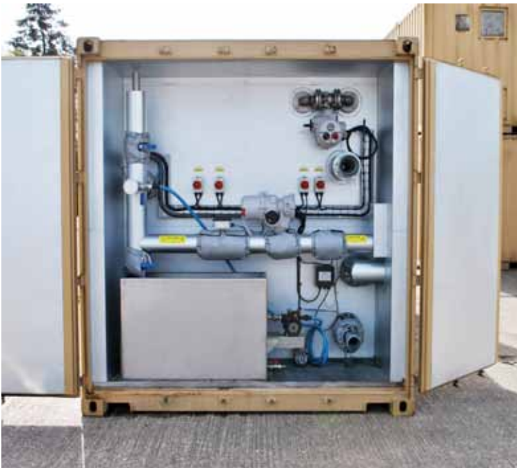
Built In Chemical Cleaning Plant Tank
