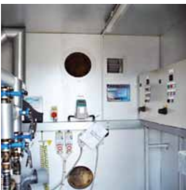
Electrical Control Room
