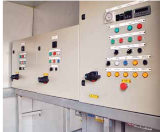
Main Control Panel with FBDA and Membrane Blower Controls
