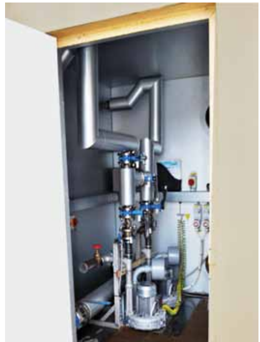
Fine Bubble Diffused Air (FBDA) and Membrane Blowers
