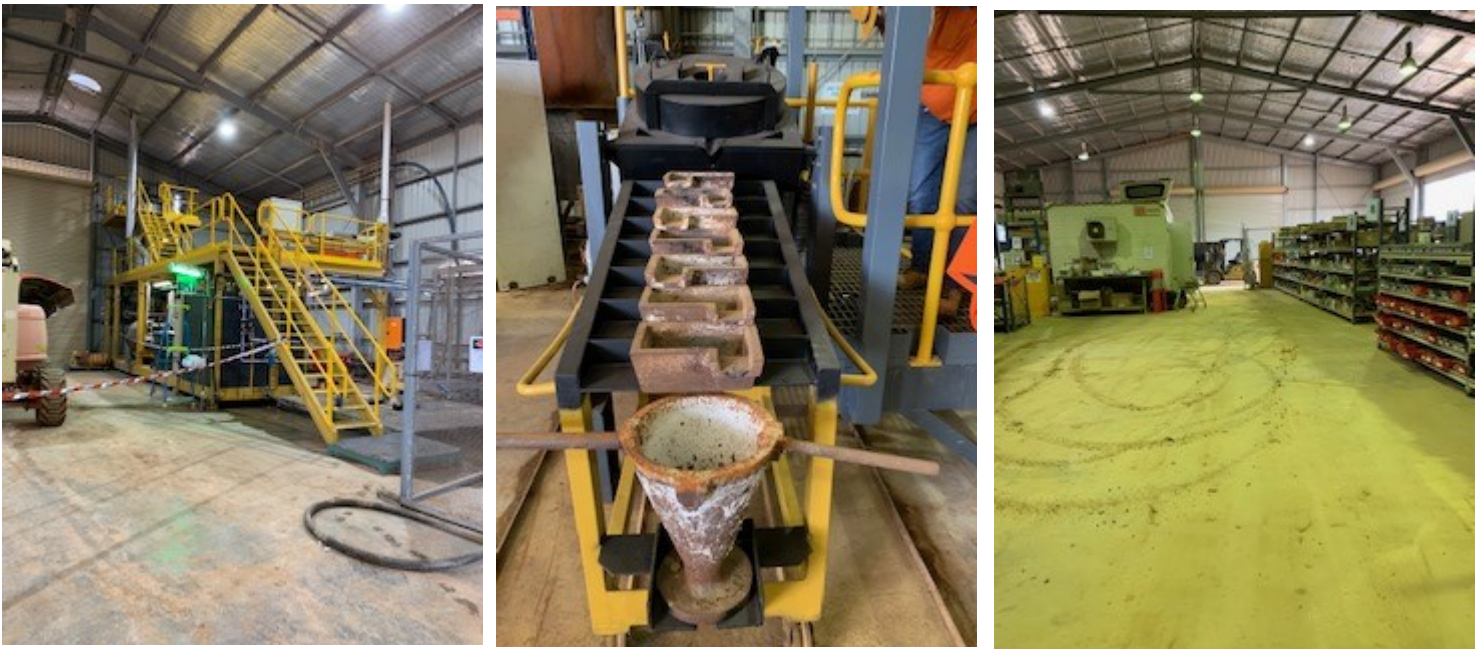
Exhibit 17 – Wonawinta plant – gold room upgrade allows on site pours, extensive spares acquired from previous owner
