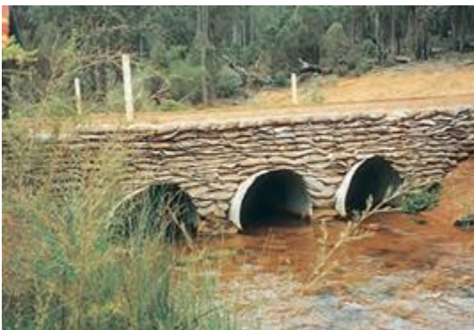
Figure A 10: Multiple culverts to adequately transfer creek flow
