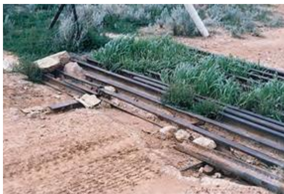
Figure 5.13: Poorly maintained cattle grid
