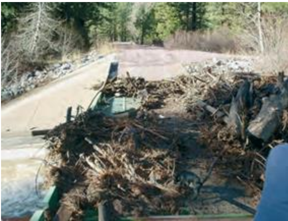
Figure 5.12: Causeway blocked with flood debris
