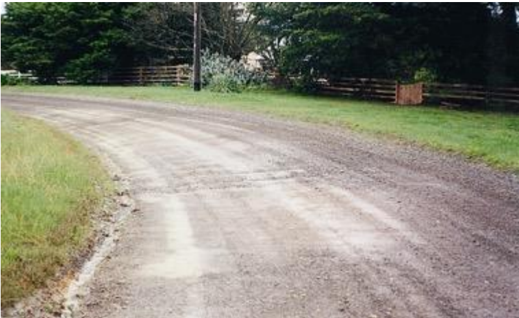
Figure 5.2: Result of poor maintenance practices on curves
