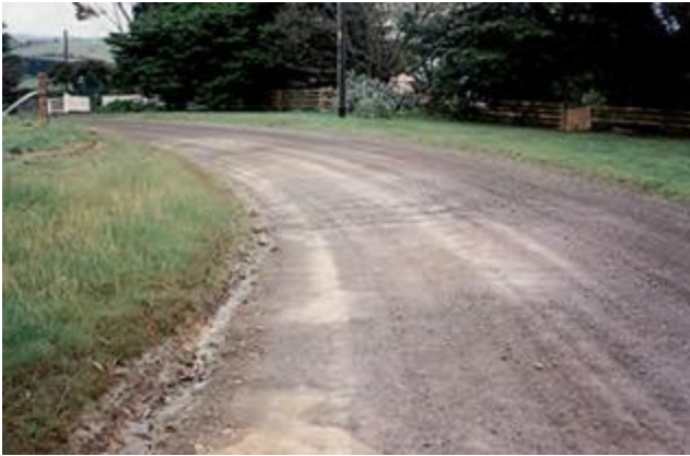
Figure D 14: Transverse scour example
