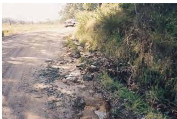
Figure 5.7: Poorly maintained table drain
