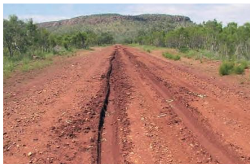
Figure 5.14: Damage due to vehicle traffic when pavement is too wet
