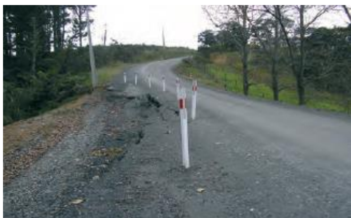
Figure D 20: Settlement of fill embankment
