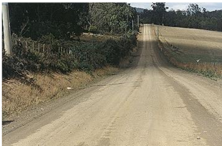
Figure C 26: Road showing the three wheeled track effect
