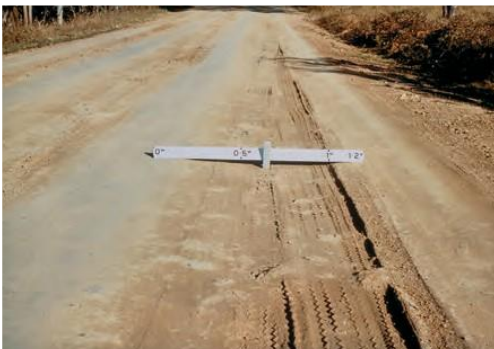
Figure D 11: Rutting in road surface
