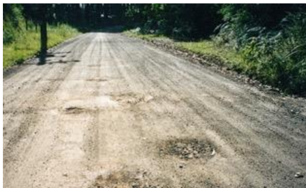
Figure D 9: Typical road where crossfall is too low (< 3% crossfall)
