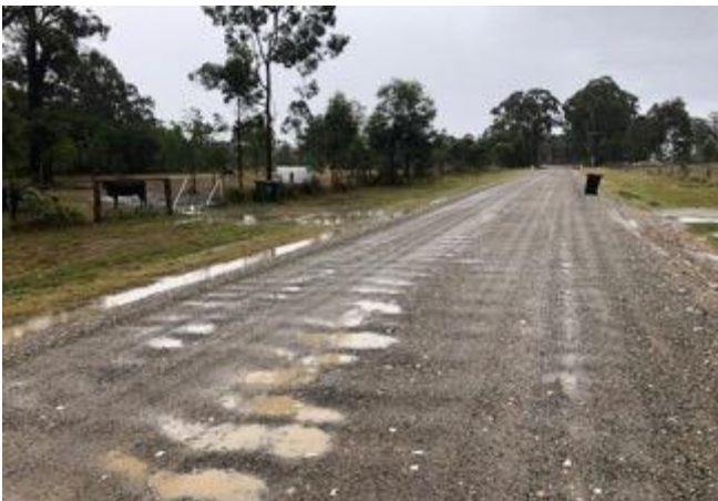
Figure D 7: Corrugations in gravel surface
