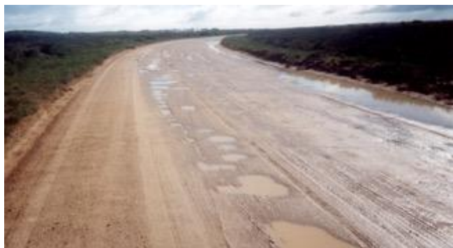
Figure C 32: Flat roads are most prone to potholes forming
