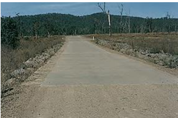
Figure A 13: A paved ford crossing with scour protection on downstream edge
