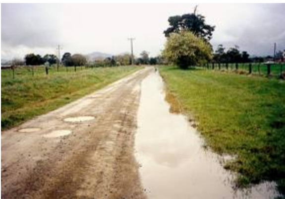
Figure 5.9: Excess water on the roadway
