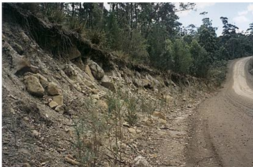
Figure C 43: Example of a badly eroded cut batter without catch drains/banks
