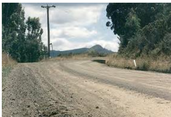
Figure D 13: Loose stones on outside of curve
