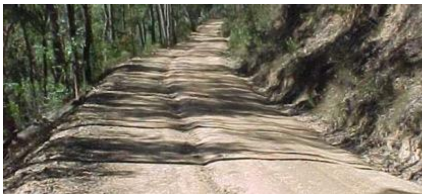
Figure C 17: Effects of steep vertical grades causing scour drains along unsealed roads
