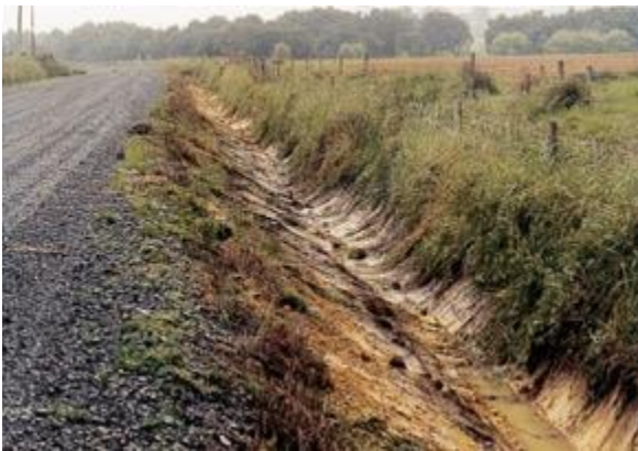
Figure 5.8: Well maintained drains but needing guide posts to delineate roadway edge
