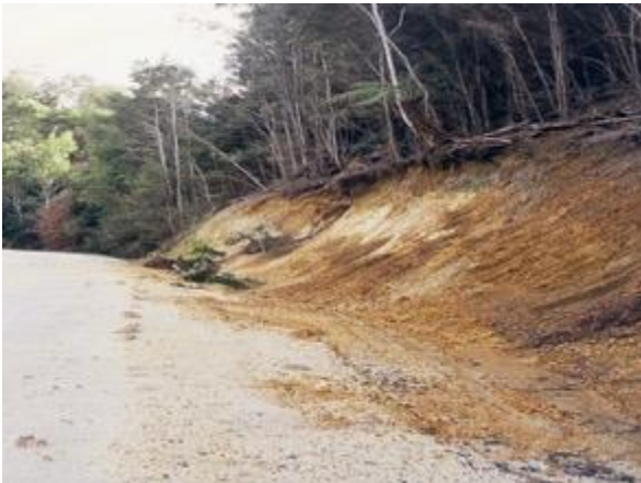
Figure A 29: Unprotected batter slope
