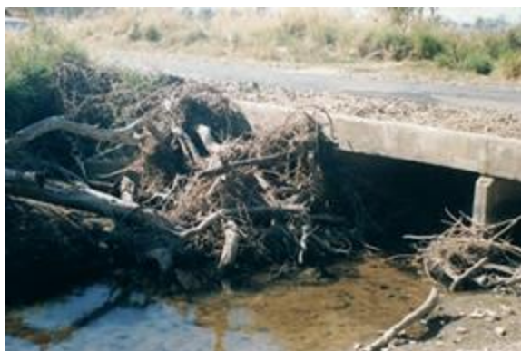
Figure 5.11: Debris collected at culvert after heavy rainfall
