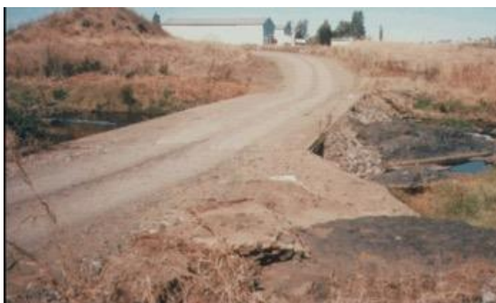
Example of a poor causeway with a lack of safety provisions, including causeway signs on approaches, guide posts and depth gauge
