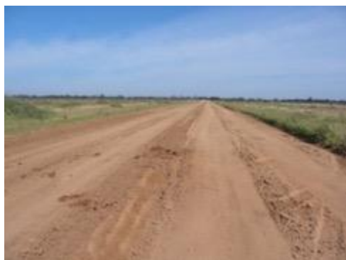
Figure D 1: Loose surface materials
