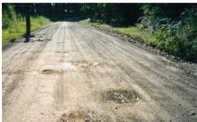
Figure 5.6: Potholes and rutting due to low crossfalls
