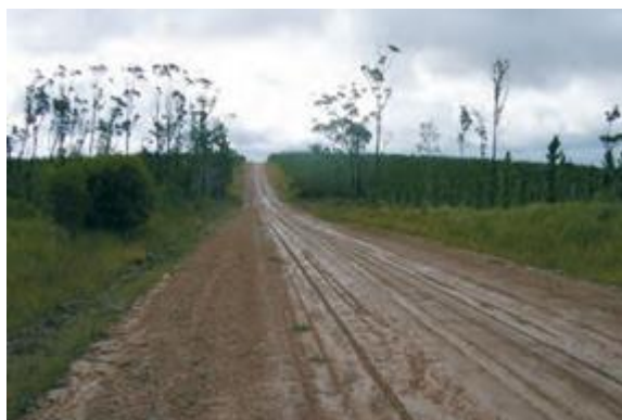
Figure D 12: Slippery surface
