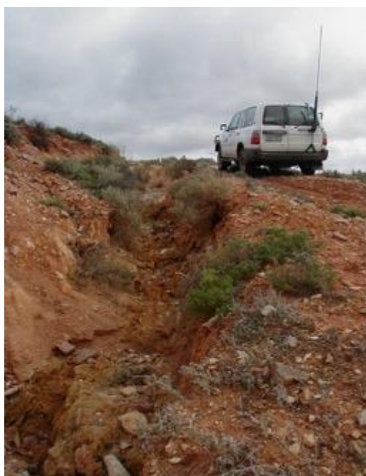
Figure 3.10: Poor location of a track on a steep grade leading to major erosion
