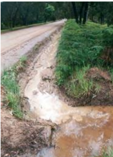
Figure A 17: Sediment laden water entering waterway from table drain
