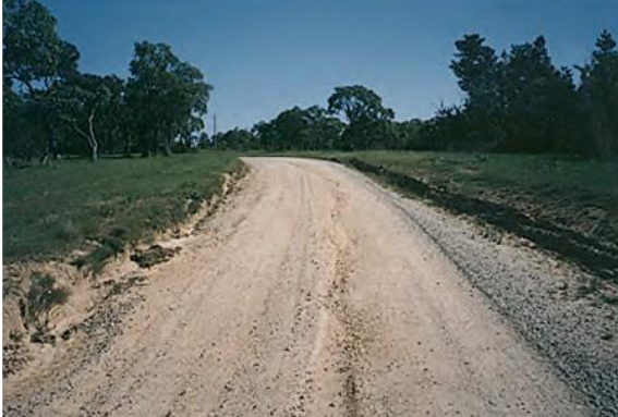
Figure D 15: Longitudinal scour
