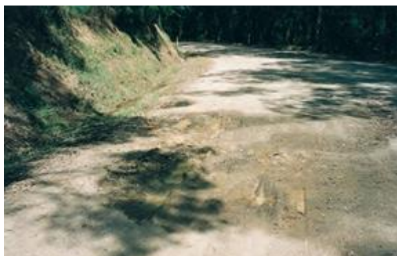
Figure D 19: Wet spot that needs subsoil drain
