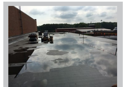
Example of a commercial roof that needs repairs
