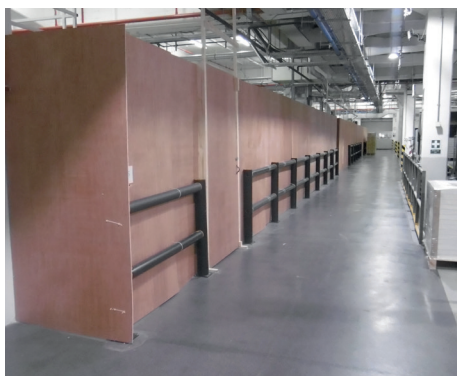
An example of a temporary wall to segregate an area of a factory and improve social distancing.
