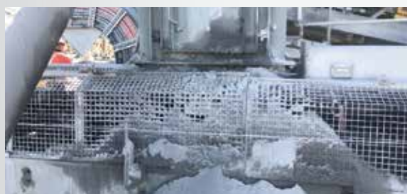
Skirt damage and spillage issues with previous system
