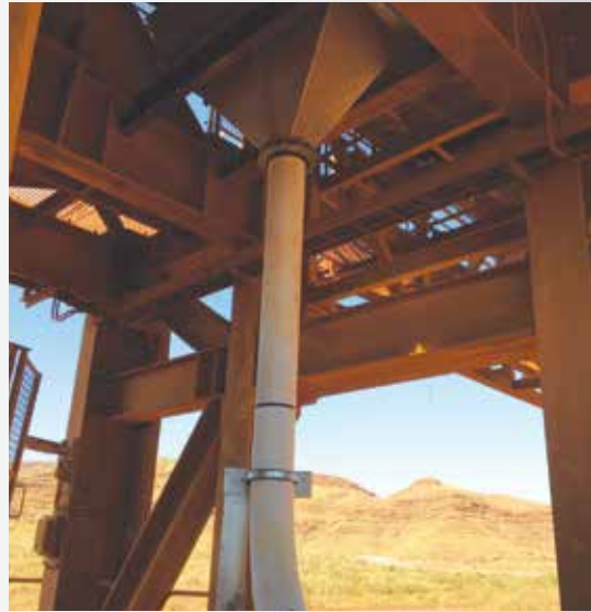
Charge Pipe Leading to Sump
